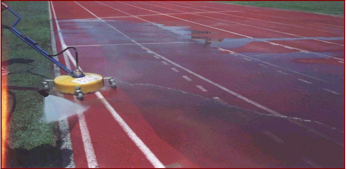
Washing of track to be done with rotary cleaning head & hand held pressure cleaner
